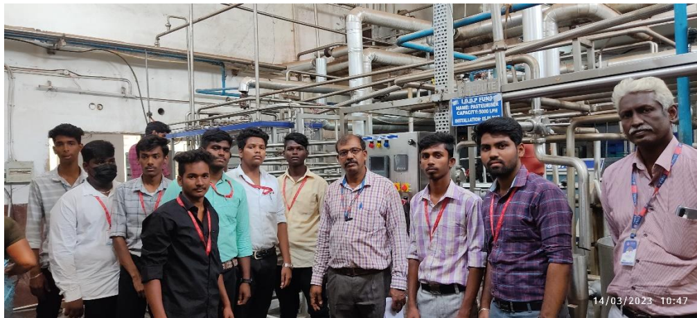
Images showing that Industries Visited by Students Aavin Milk Dairy Plant located at Nanjikottai Road, Thanjavur
